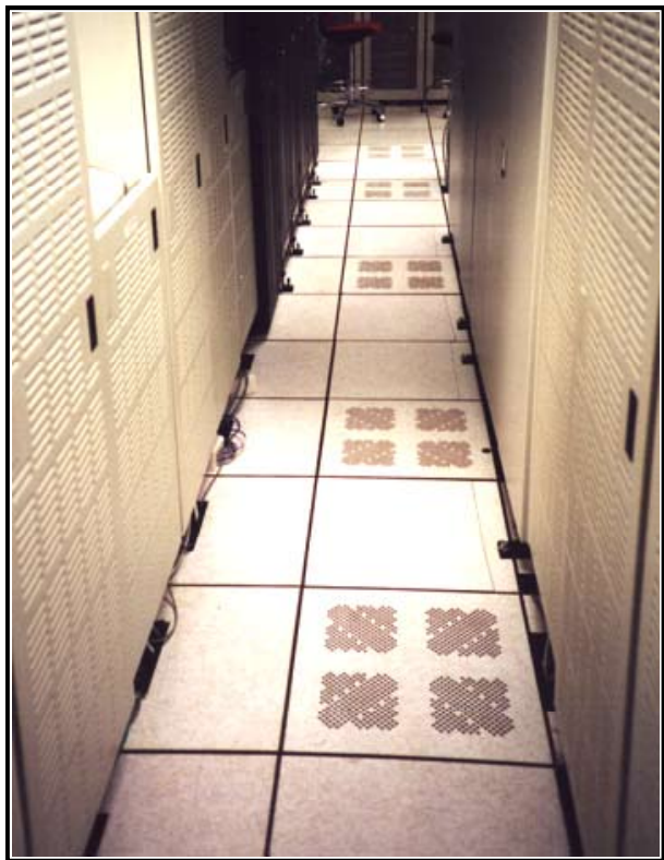
Figure 3. These misplaced perforated tiles and less obvious unmanaged cable openings are allowing valuable cold air to escape. Forty-five percent of the capacity of a 20-ton cooling unit is being wasted in this picture.
